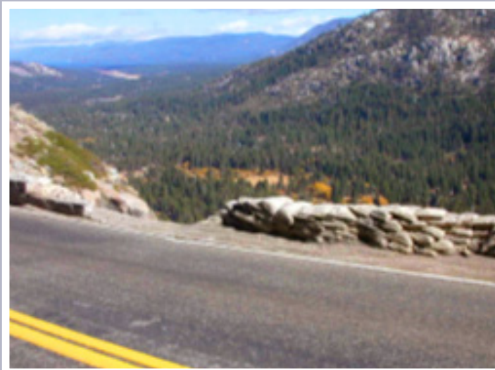
Damage at south end of Johnson Pass Sidehill (Caltrans 2006)
