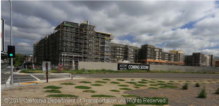
High Density Housing under construction, near westbound SR 85 at Cottle Road off-ramp
