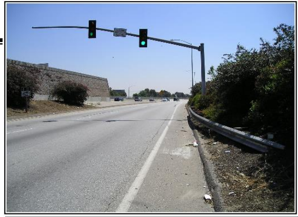
Ramp Meter Signal Lights
