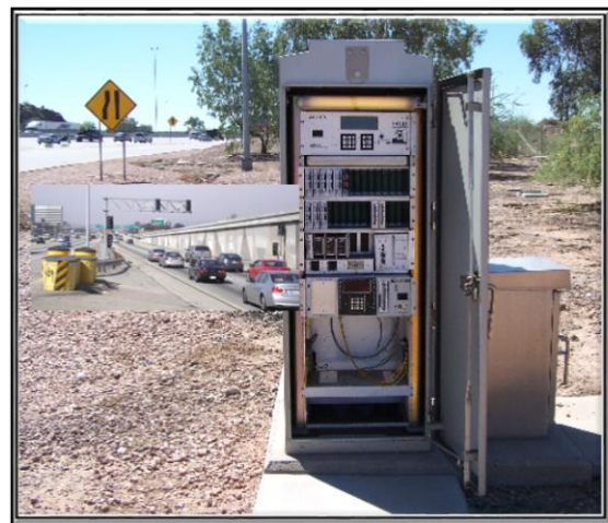
Ramp Meter Controller/Cabinet
