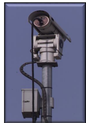
Close Circuit TV (CCTV)
