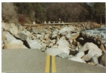
Route 140 damaged by the 1997 storm disaster (1997 photo)
