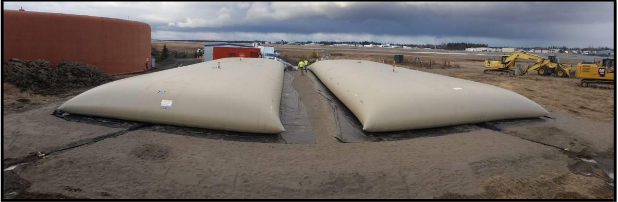
Figure 11. Two 100,000 gallon water storage bladders on a construction site. ( https://readycontainment.com/bladder-tank-gallery/ )
