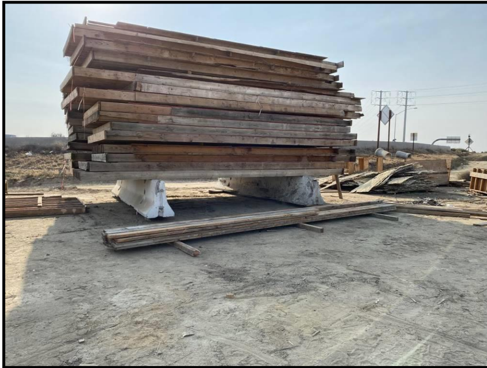
Figure 6. Construction materials placed up on K-rails on the Centennial Corridor road construction site in Bakersfield, CA. (Photo by E. Noel)
