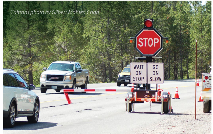
Remote-operated flagging devices such as this one on State Route 89 perform the same work as humans without exposing them to traffic.
