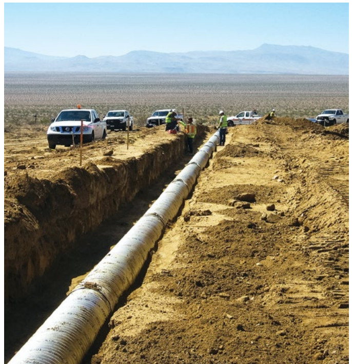
A pipeline to route water from the highway is installed as part of the Freeman Gulch project. The desert area is prone to flash flooding.
