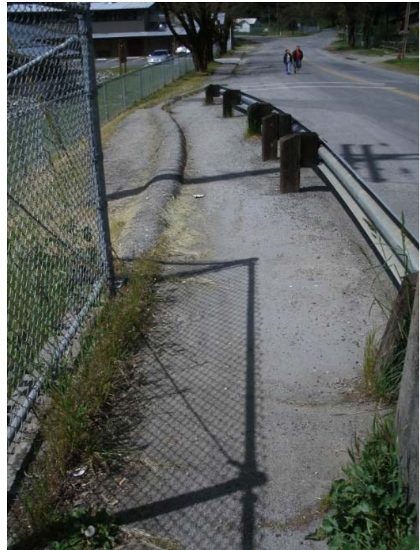
Figure 20: 2nd Street Bridge is non-ADA Compliant (Source: Middle Klamath River Community Transportation Plan , Lumos & Associates for the Karuk Tribe)
