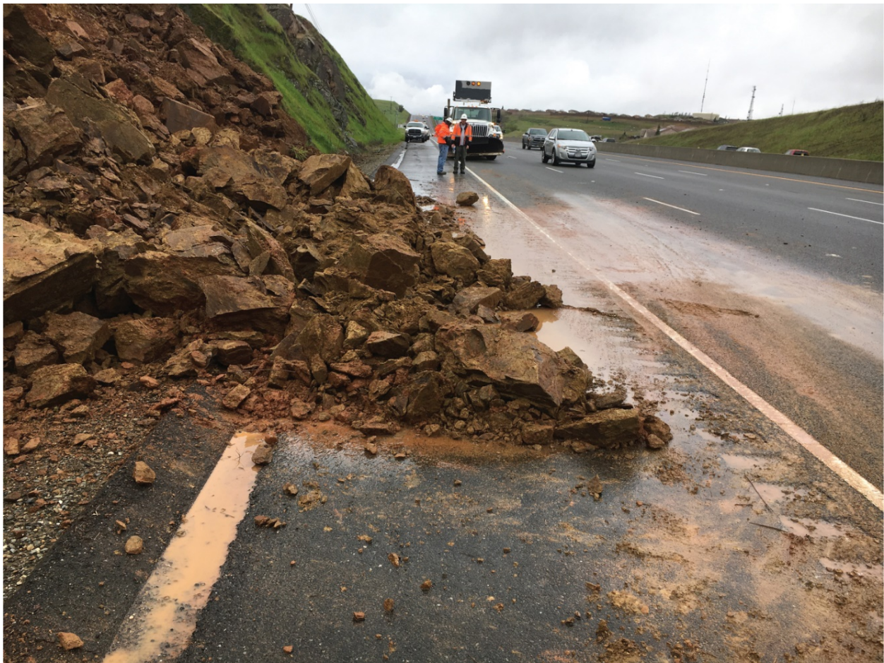
MUDSLIDE NEAR LATROBE ROAD, EL DORADO HILLS
