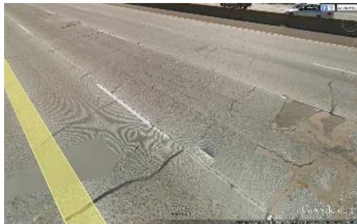
DAMAGED PAVEMENT SLABS SOUTH OF SUTTERVILLE
