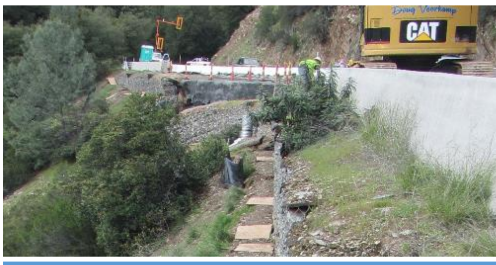
GABION WALL SLIDE
