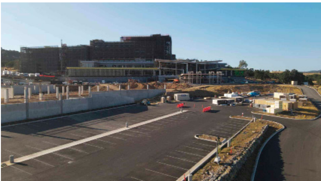
The new Chicken Ranch Casino and Resort is currently under construction in Jamestown.
